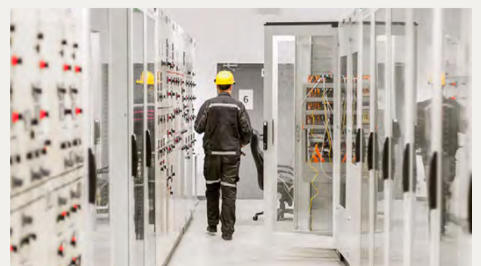
Electrical switching rooms
